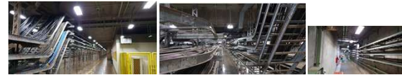
The cable trays are of ladder type and are manufactured from hot dipped galvanized steel
